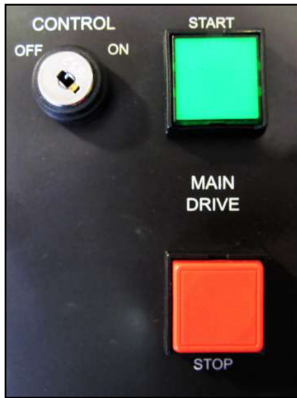
FIGURE 6-3 Control ON-OFF Keyswitch and Main Drive START-STOP Pushbuttons
